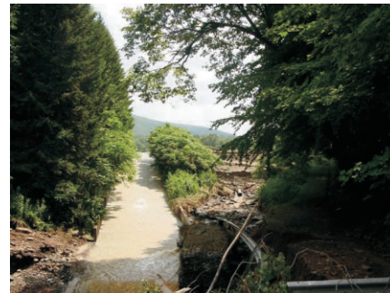
Spillway from reservoir. Note remnant of original transmission main at lower center. 450' of new piping was needed to close the breach. Photo courtesy of Chatfield Engineers
