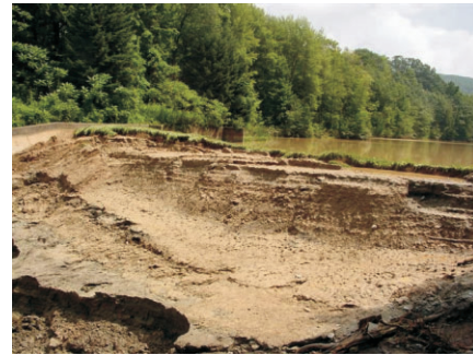
Erosion of the original dyke. Photo courtesy of Chatfield Engineers
