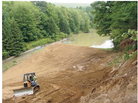
A view of UTT's speedy restoration of the reservoir dike. Photo courtesy of Chatfield Engineers
