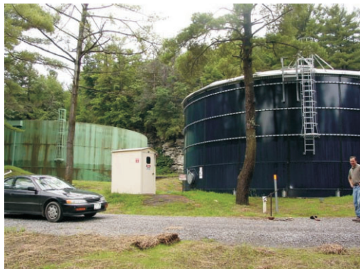
Village storage tanks for treated water. Look closely to see remaining levels at condensation lines: At ladder bottom on the green tank and up three rungs of the ladder on the blue tank. Conservation was a major concern! Photo courtesy of Chatfield Engineers
