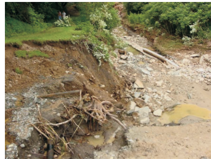
Erosion from flash flood. Note pipe remnants at right and at lower left. Photo courtesy of Chatfield Engineers
