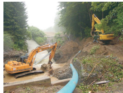
A giant hole was washed out (now filled with stone) where UTT's Case Excavator now sets. Originally the cast iron main was routed through here, now replaced with 12" polyethylene pipe. Photo courtesy of Chatfield Engineers
