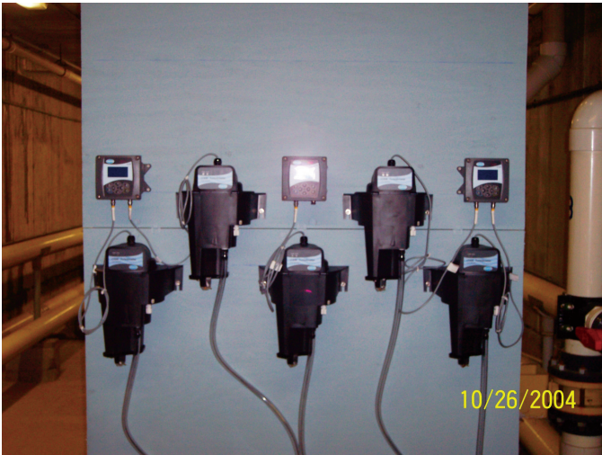
Part of Hach Equipment Being installed purchased with Grant Funds
